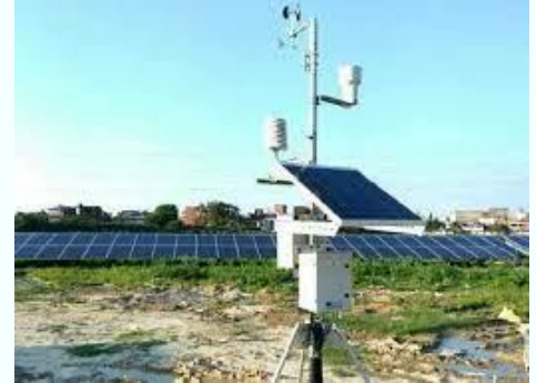
Automatic Weather Station in Pakistan
